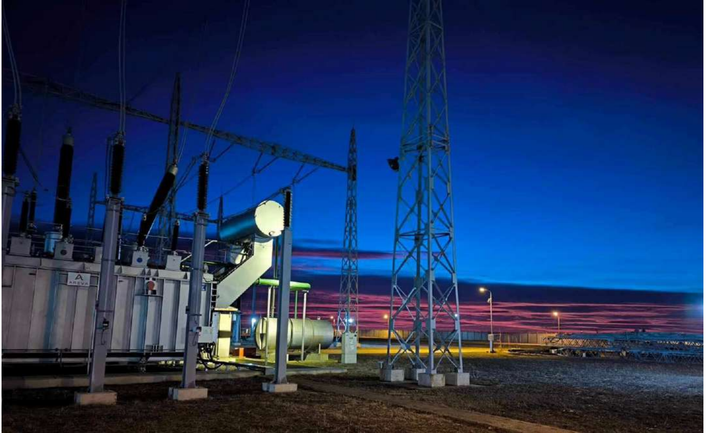
Tariverde 400.110 kV station
