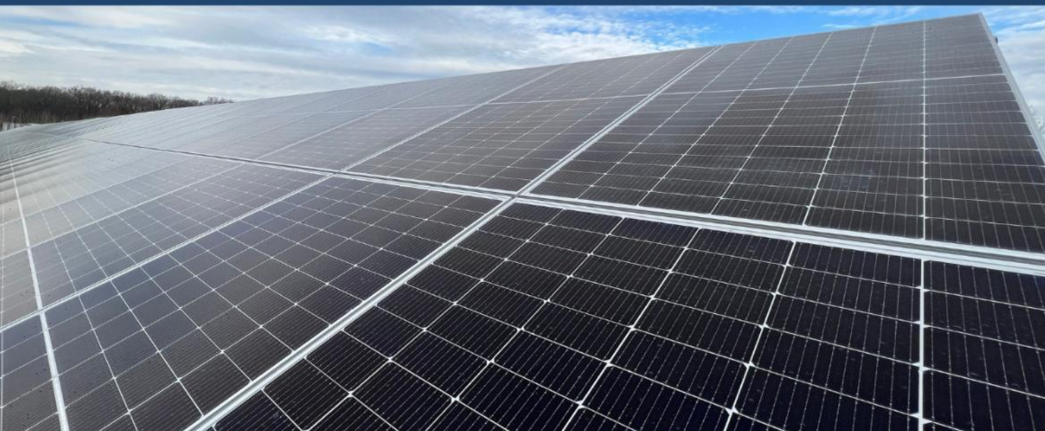
Premier Energy's 1.9 MW solar park, located in Prahova County, Romania.
